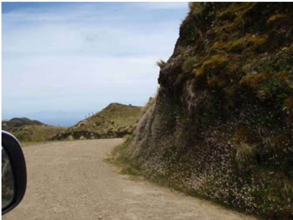
PHOTO 39 - 2m cut back required on RHS of main track for truck access (Building at top of cut)
