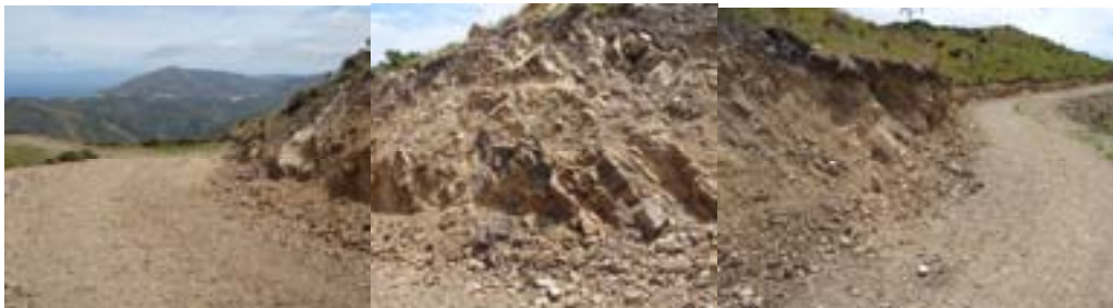
PHOTO 27 to 29 – Corner to be cut back by 3 to 5m for truck access
