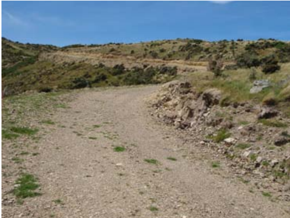
PHOTO 36 – 1m cut back required on RHS of main track for truck access
