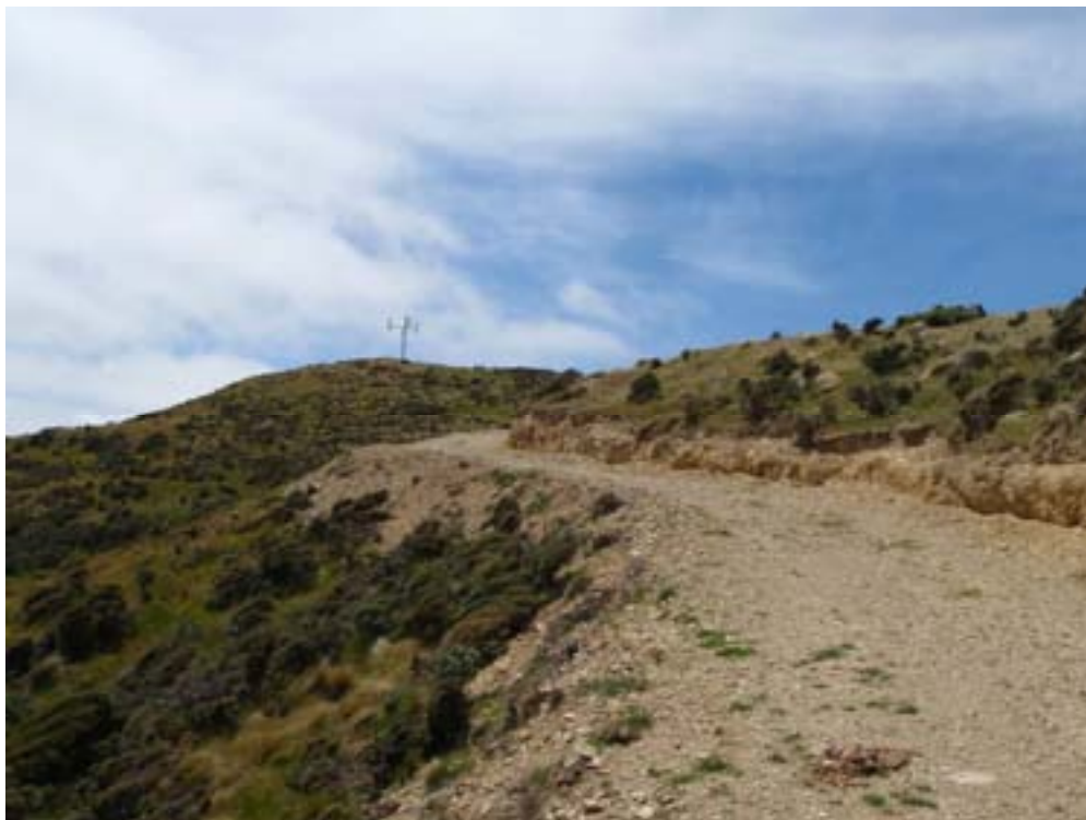
PHOTO 37 – 1m cut back required on RHS of main track for truck access
