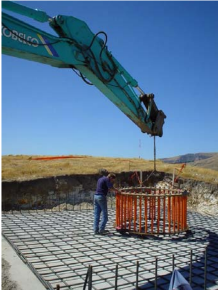
The foundation prior to pouring the concrete, showing the reinforcing and holding down bolts ....
